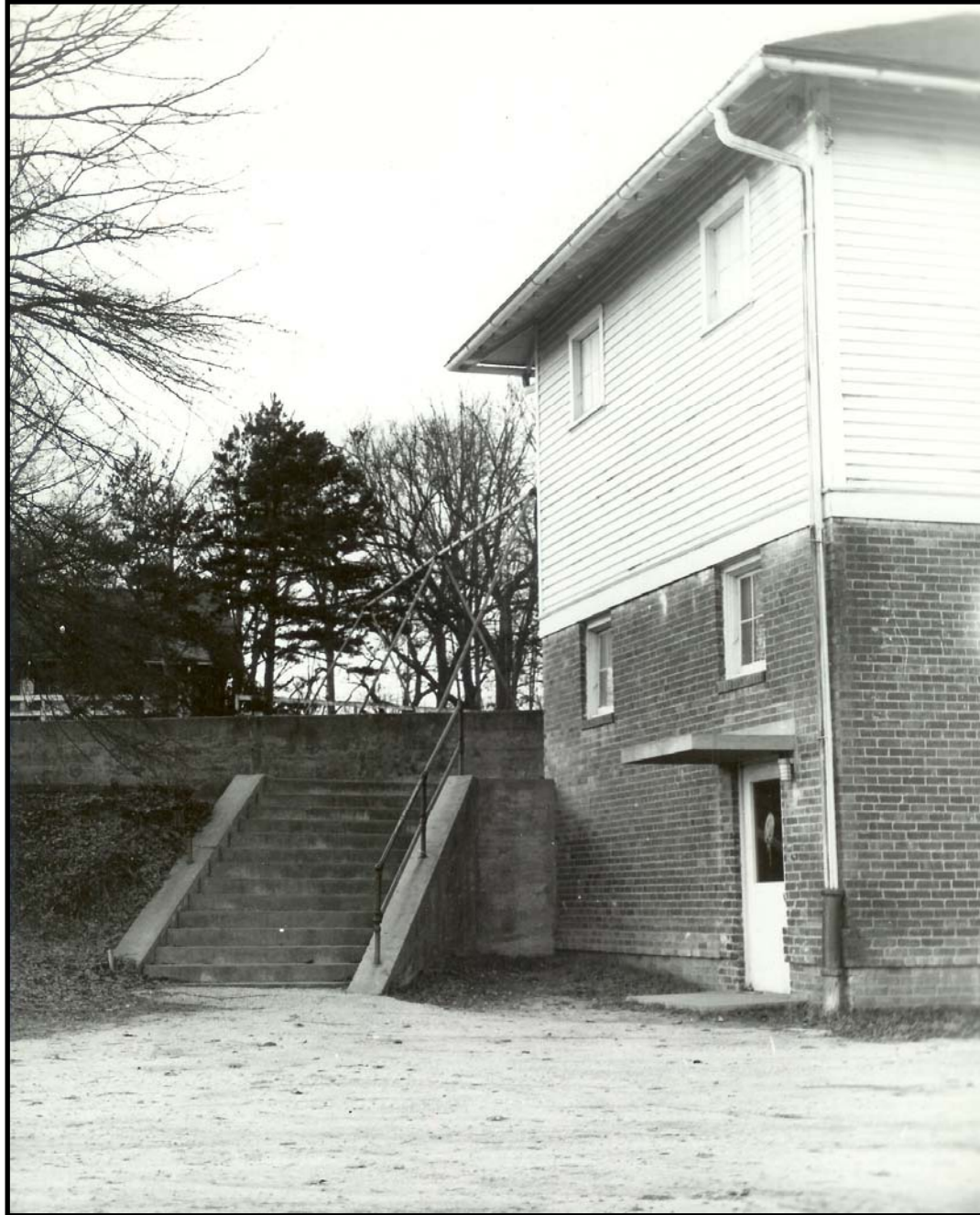
This view is of the steps that come down from the playground behind the Annex to the level of the school cafeteria.
